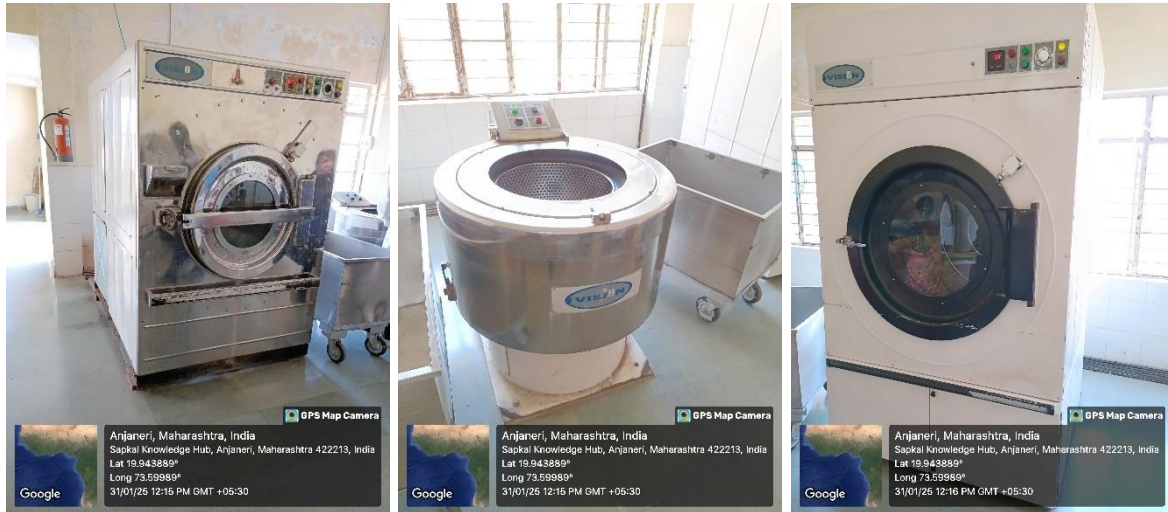
Geotagged photo of washing machines installed in the laundry of the institute
