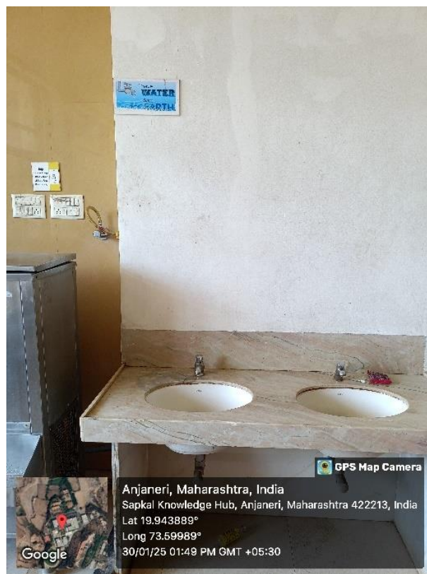
Geotagged photo of low flow faucets for hand wash and water conservation awareness poster in canteen
