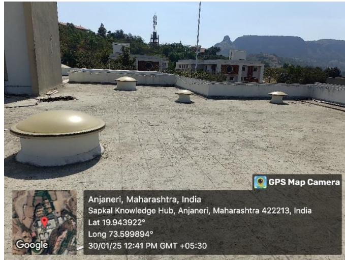
Geotagged photo of light ducts provided in the building
