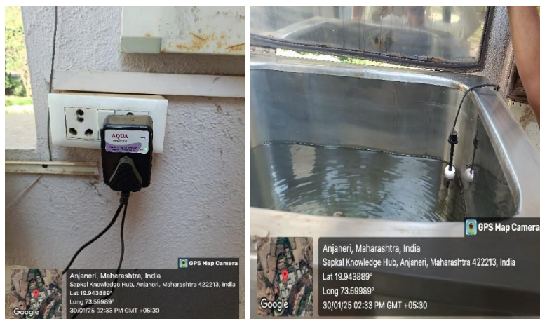
Geotagged photo of water level controller installed in RO unit
