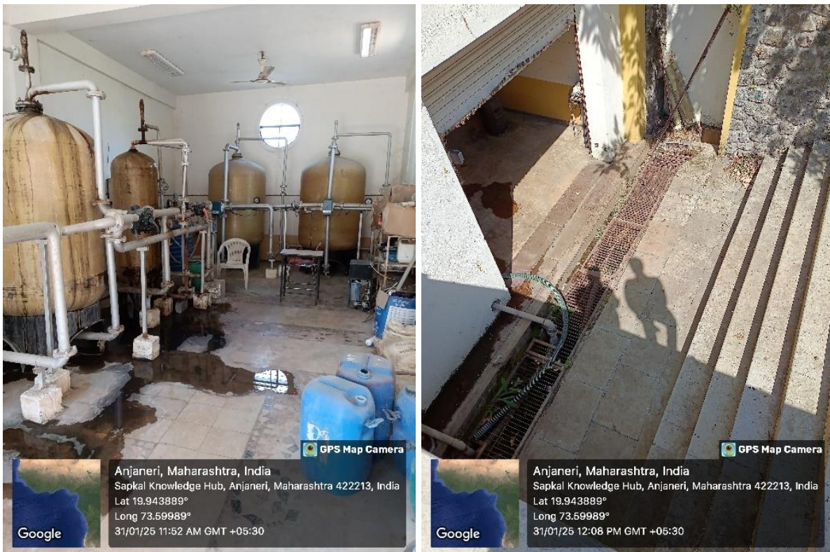
Geotagged photo of RO Water purifier installed and reject water channel
